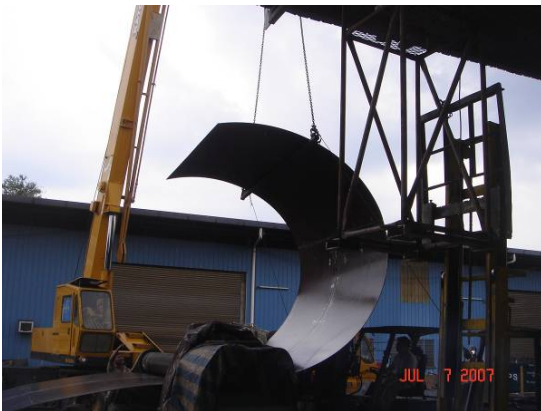
Ducting for bending
